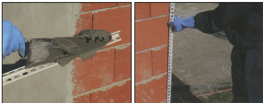
Fig. 3.39 Application of a perforated PVC protection profile in a salient corner of a wall [35]
