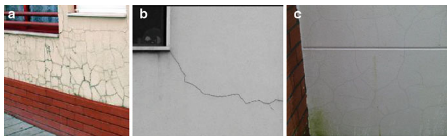
Fig. 2.30 (a) Mapped cracking/fissures; (b) oriented cracking in traditional render [71]; (c) cracking in pre-dosed render [65]
