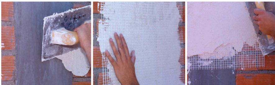
Fig. 2.18 Application sequence of a glass fibre net in the transition zone between a concrete column and a brick masonry wall [64]
