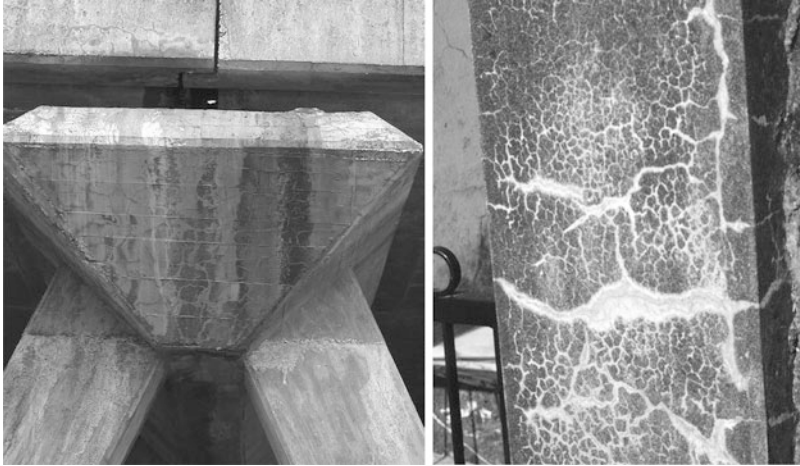
Fig. 4.15 Cracking caused by alkali-silica reactions
