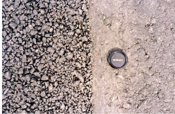
Fig. 5.7 Texture of the pavement surface in porous asphalt ( left ) and asphalt concrete ( right )
