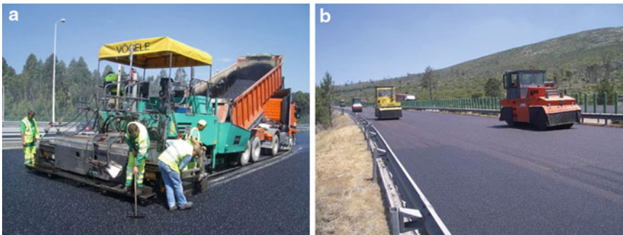
Fig. 5.9 Pavement construction: (a) asphalt paver; (b) rollers operating the bituminous mixture compaction
