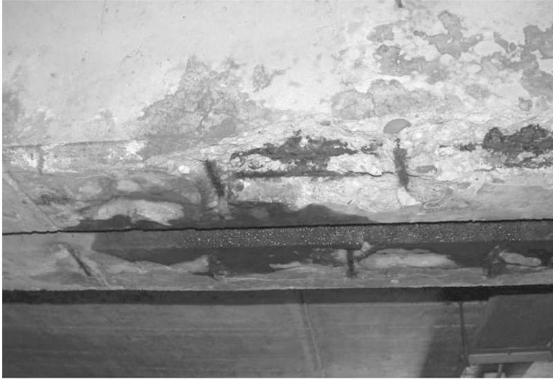
Fig. 4.14 Concrete degradation due to corrosion of reinforcements
