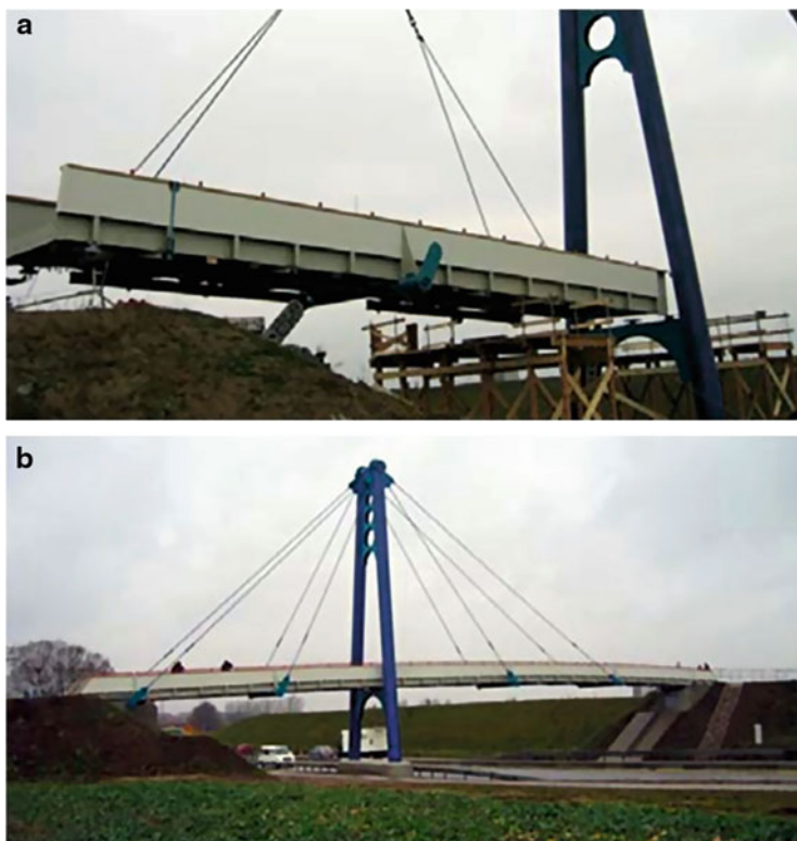
Fig. 16.1 Pedestrian Bridge in Schwerin, Germany. A two-component epoxy structural adhesive was used in this bridge to bond prefabricated elements of GFRP (glass fibre-reinforced polymer composite having an unsaturated polyester resin matrix) constituting the segments used in the bridge deck [4]
