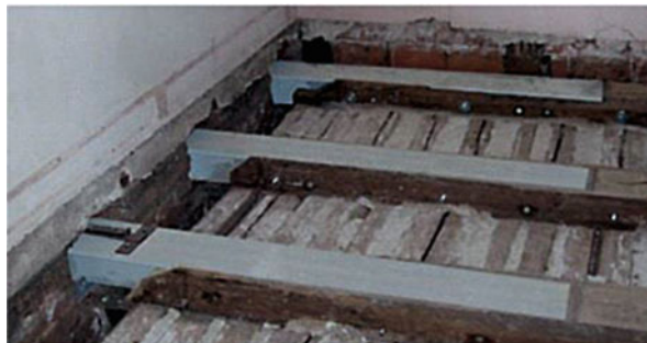
Fig. 11.30 Use of GFRP pultruded profiles in the rehabilitation of a degraded timber floor [32]
