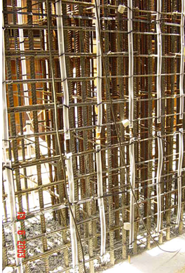
Fig. 15.22 Installation of a cathodic protection system in a structure during construction stage (courtesy of ZetaCorr)
