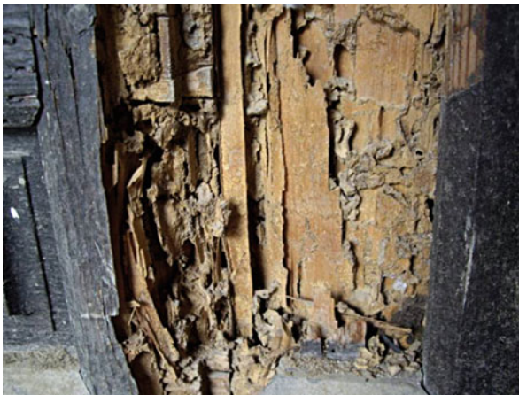
Fig. 12.11 Laminated appearance of the wood and the presence of mud tunnels resulting from the action of subterranean termites
